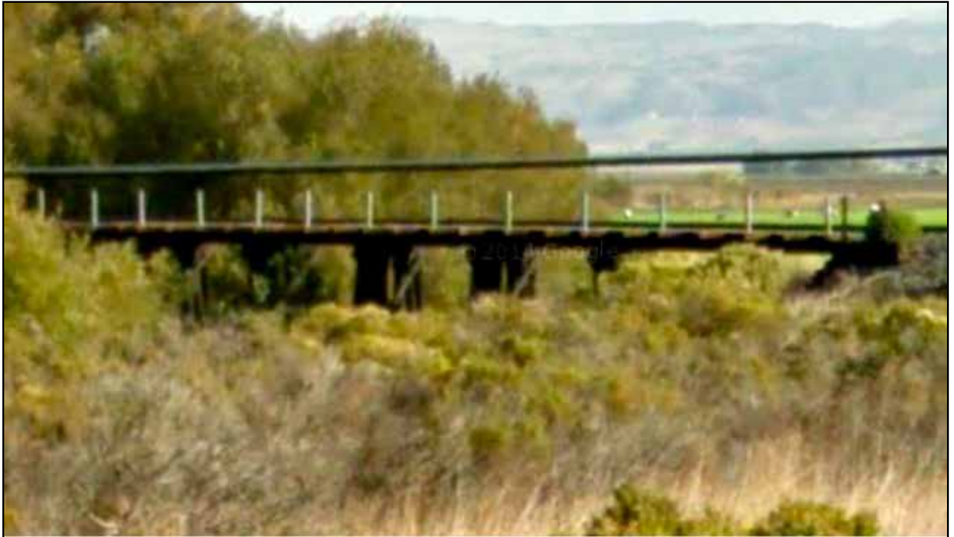
Figure 12. Southern Pacific (now Union Pacific Railroad) pile-bent trestle over Pajaro River, near San Benito County line, and on active railroad line.
